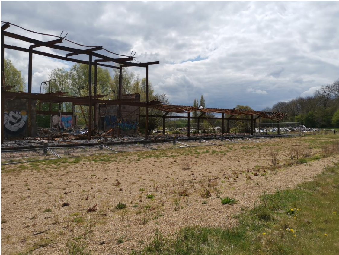
Above/Below: Former front elevation of the remaining structure from the northern side of the site
